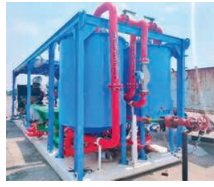
Sewage Treatment Unit
